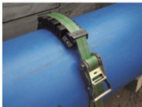
FIXBLOC is held on the pipe during fusion using a 50mm wide standard tensioning belt.
